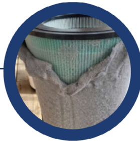
Filter After 2 Years No Maintenance
